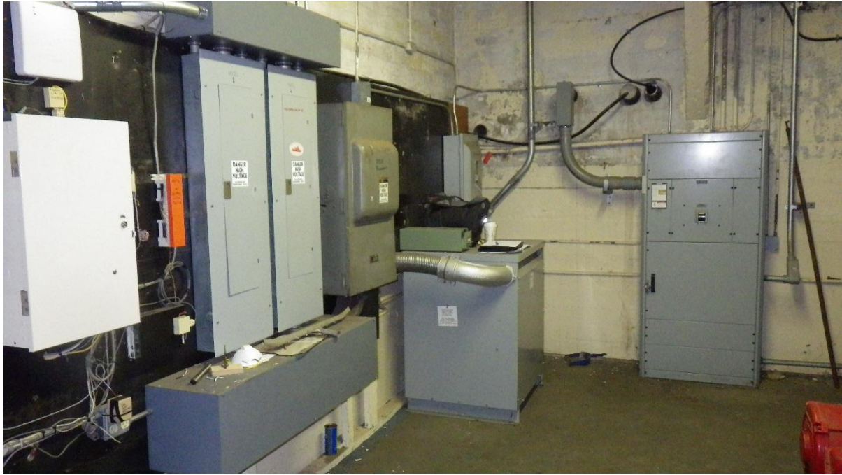
Electrical Service Entrance
