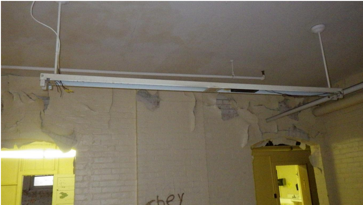
Typical Lighting Fixtures
