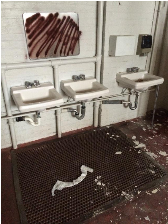
Typical Plumbing Fixtures
