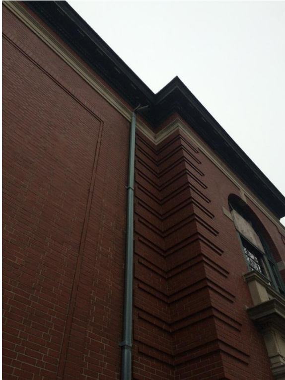
Typical Damaged Downspout
