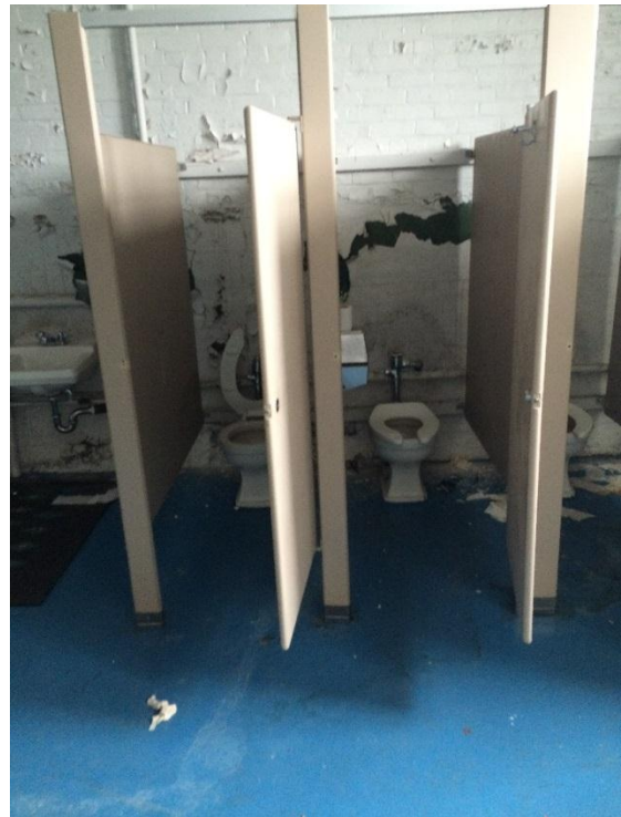
Typical Plumbing Fixtures
