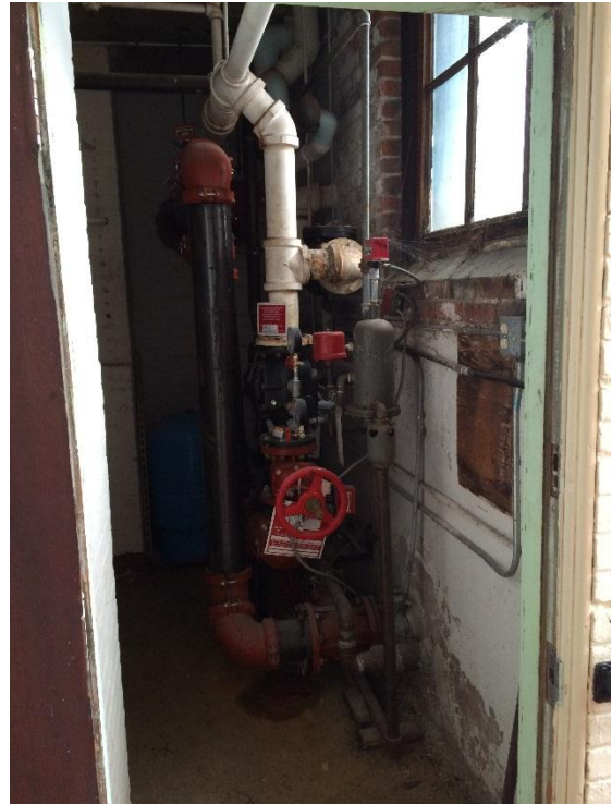
Water and Fire Protection Service Entrance
