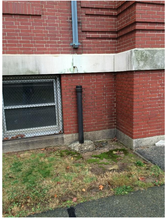
Typical Damaged Downspout
