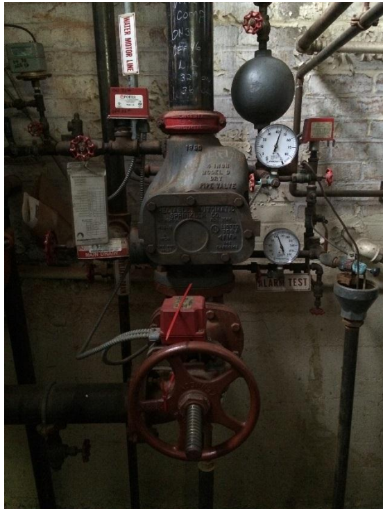
Dry Pipe Alarm Valve
