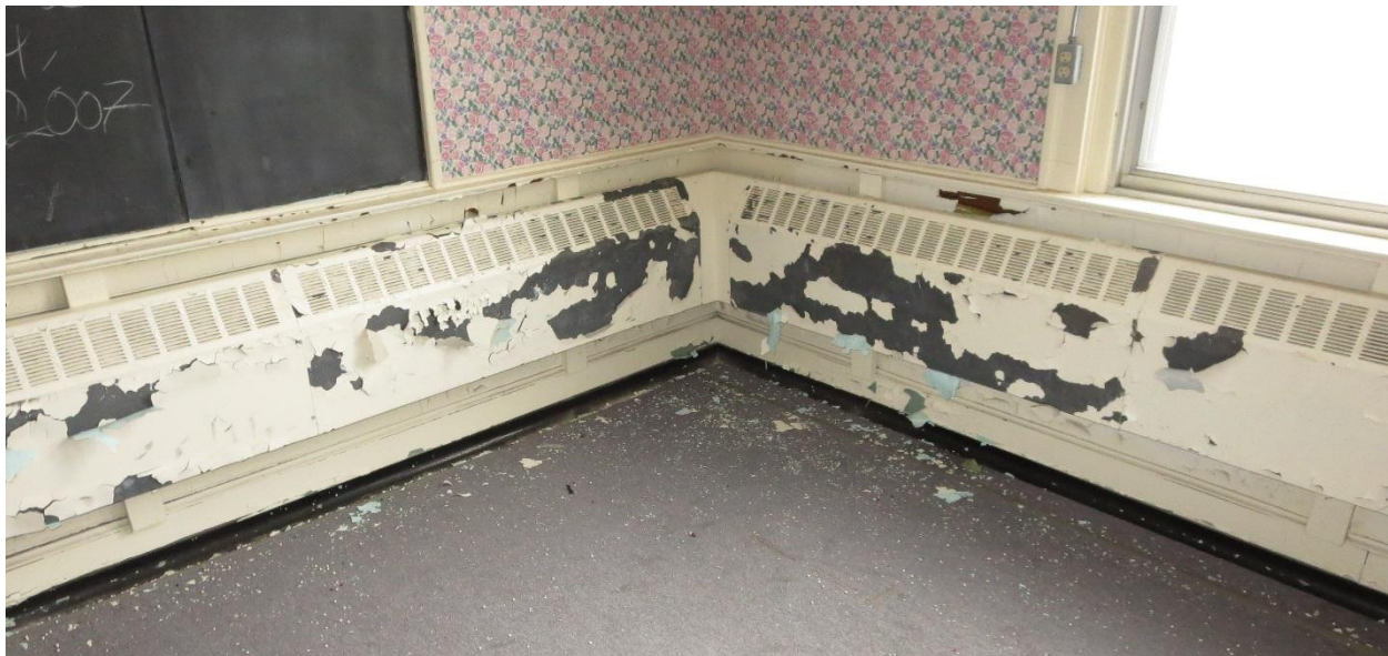
Typical Steam Perimeter Finned Tube Radiation
